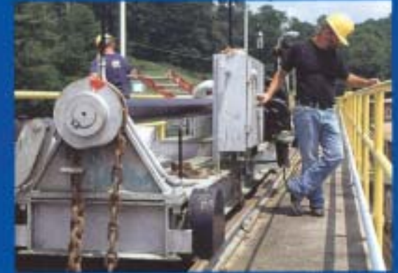
Maintenance personnel operate the Tainter Gate Hoist which regulates the lake elevation.
