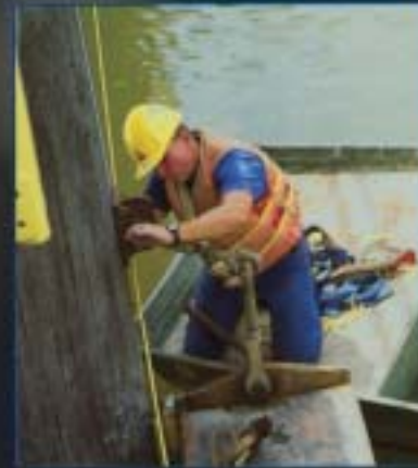
An employee inspects and performs maintenance on the Tainter Gate. (Below) The plant equipment is kept clean.
