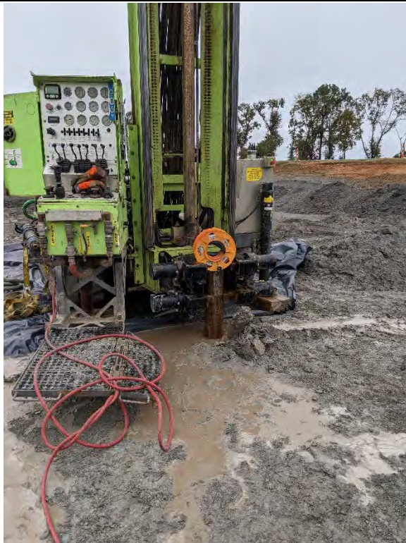
Two-inch inner casing of well overdrilled with 6 inch auger down to 53 ft.
