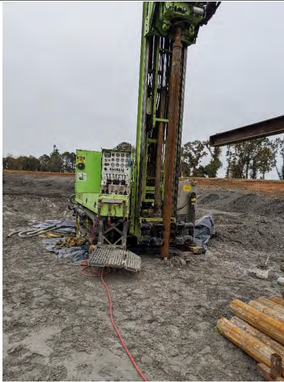
Setup drill rig on well to begin overdrilling well to abandon well.
