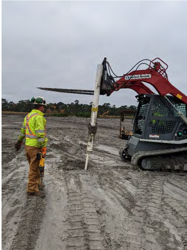
Removal of riser pipe and outer casing above ground surface, 6 ft 9 inches.
