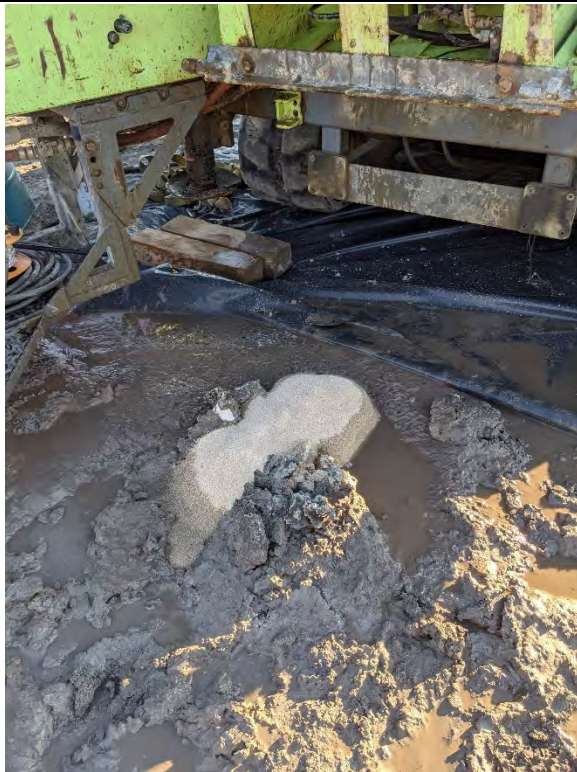
Finished backfilling 25 ft, 9-inch borehole from bottom of ash pond to ground surface.
