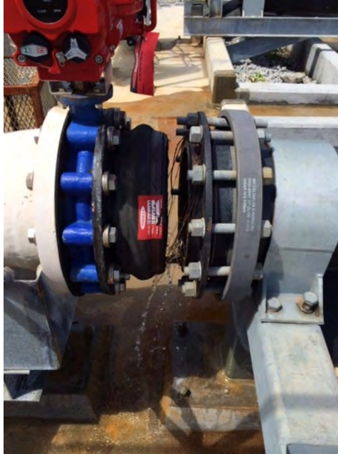
Exhibit 1 Expansion Joint Rupture of the Return Water Pipe
