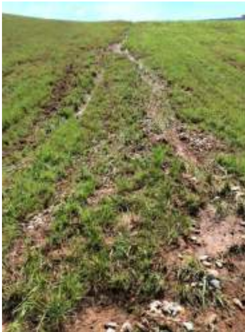
Exhibit 2 Vegetative Cover on the Embankment Northeast (Downhill) of the Return Water Pipe Rupture
