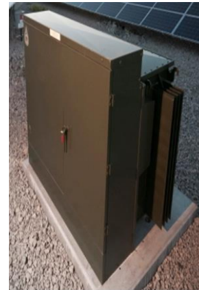
Three Phase Padmount Transformer
