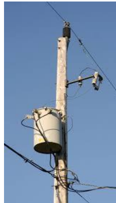
Single phase line & transformer
